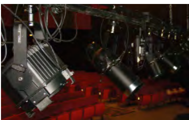
In the auditorium new state-of-the-art LED theatrical lighting has been installed.
